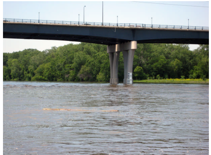
(above) High water last year reduced clearance at the I 35E bridge and sent large logs downstream
