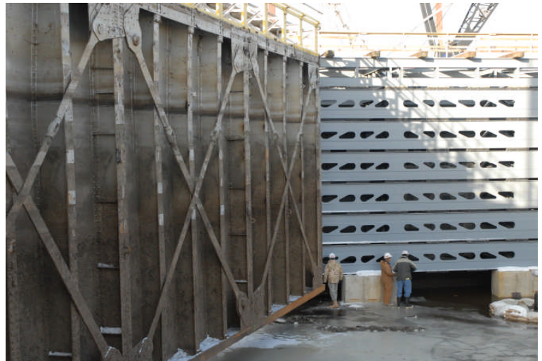
Above: Lock and Dam 3 was dewatered and the walls and gates were refurbished in early 2008.
