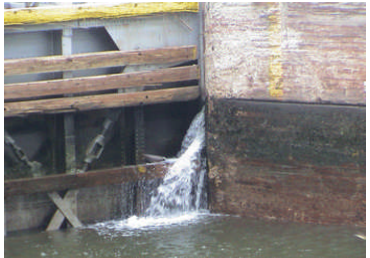
Above: The Waterways Council uses this picture of the Emsworth lock on the Ohio River to illustrate the condition of much of America's aging waterway infrastructure.
